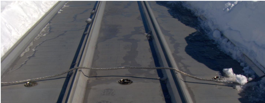
Lightning protection cable (Photo source: Zurich)
